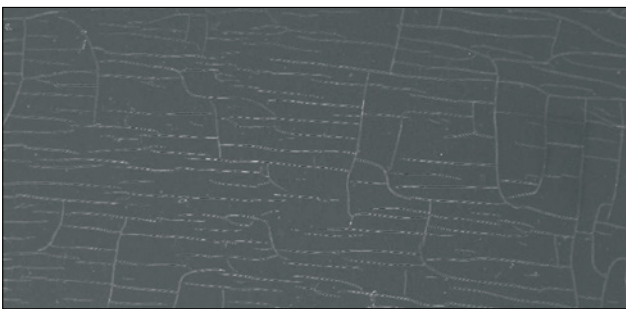
The joint has been damaged throughout by UV-radiation.
